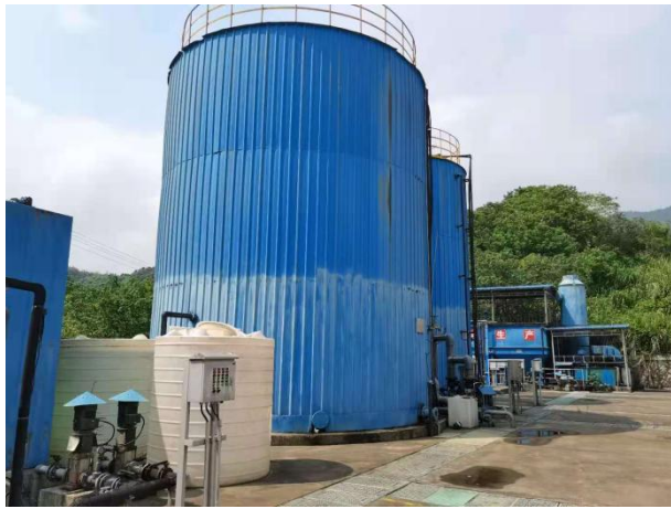
硝化罐、反硝化罐
